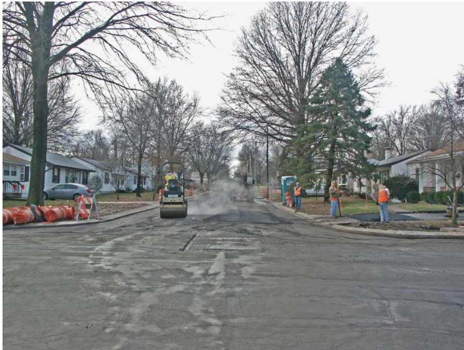
Construction began November 2009 for the Old Town Street & Storm Water Drainage Improvement Project Phase VIIA 800 Block of Clark Street.
