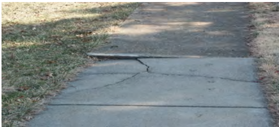
Sidewalk with trip hazard
